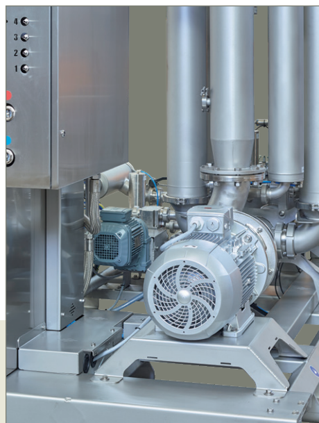
Optimal accessibility to the filtration loop
